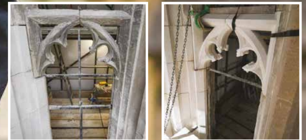
Before and after photographs of restored stone tracery in the South Nave Aisle
